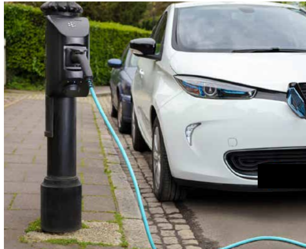
Figure 56: Example of on-street electric vehicle charging points.
