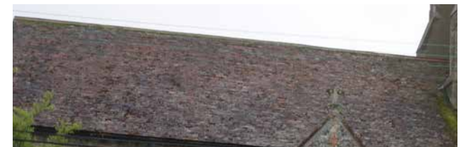
Figure 41: Local examples of roof materials that could be used in new development, e.g. grey slate and clay peg tiles.
