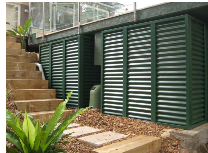
Figure 40: Concealed tanks integrated with the design.
