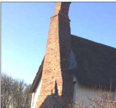
Crooked Chimney Stack
