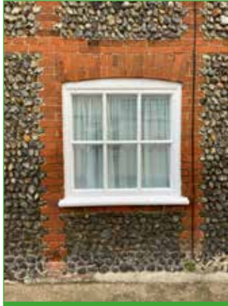
Window openings in this predominantly flint elevation have been enhanced with use of brick surround and segmented arch.
