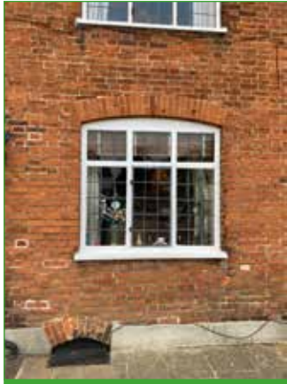
This brick facade includes the use of segmented arch to window and plinth opening.
