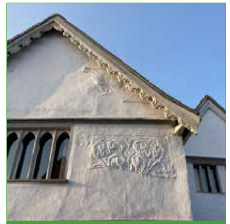
The Priory, an historic asset with generous eaves, decorative barge boards and pargetting.
