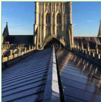
Roof-mounted photovoltaic installation on Gloucester Cathedral's south nave. Image © St Anns Gate Architects
