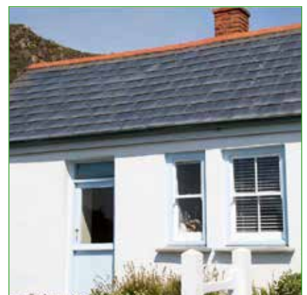
A domestic building with the existing roof covering replaced by PV slate tiles. Image © Historic England
