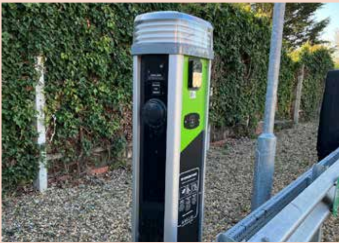
EV charging point
