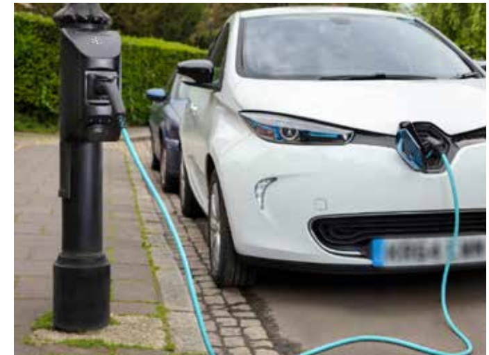
Figure 81: Public car charging point incorporated into the street design.
