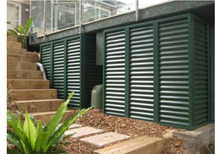
Figure 76: Concealed tanks integrated with the design.
