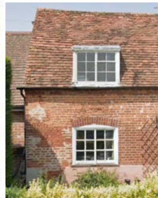
a case for some further repair and maintenance
