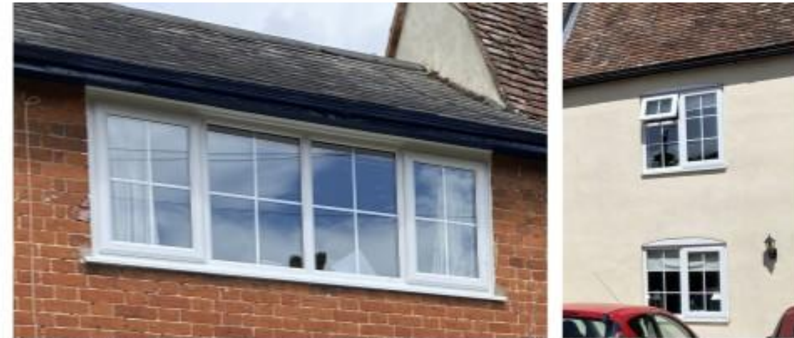
Figure 239-240: Examples of poorly detailed modern replacement windows. Flush to the surrounding walls instead of recessed, applied or 'stuck on' glazing bars' heavy opening casements overlapping instead of flush with the surrounding frames, material not confirmed but potentially plastic or aluminium
