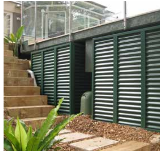
Examples of concealed tanks used for rainwater harvesting
