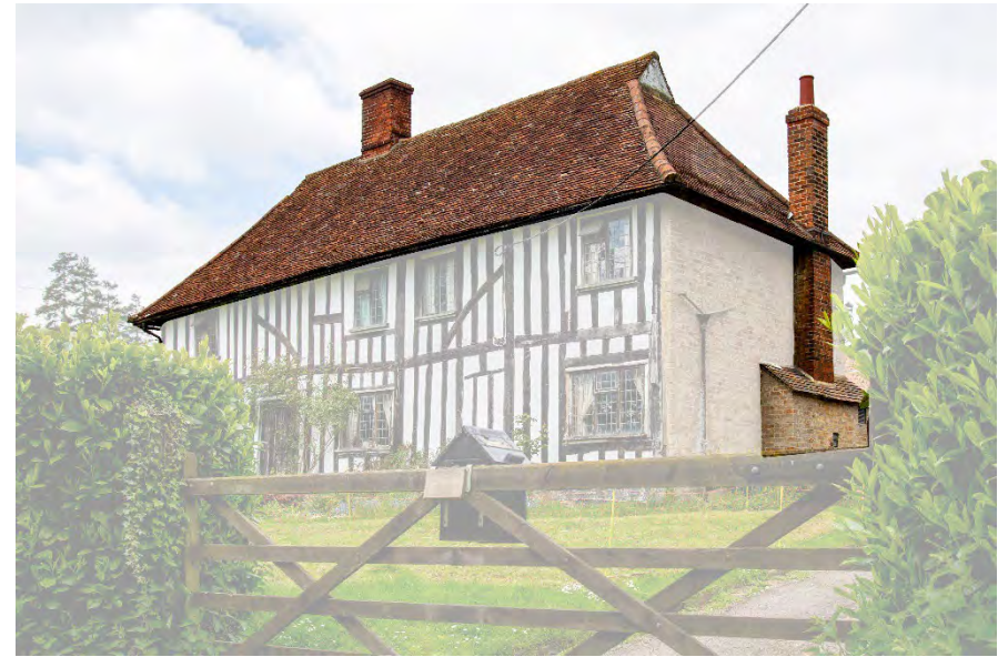
Pound Farmhouse, example of a hipped tiled roof with north and south ends with gables and a ridge chimney stack.
