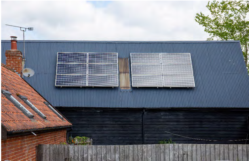
Potash Farm, Old School Road with solar panels.
