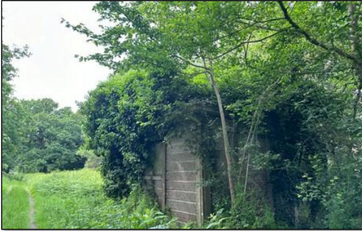
figure 108: Former railway platelayer hut in a poor state of repair.
