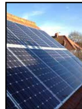
Restrict overshadowing from neighbouring properties onto the panels
