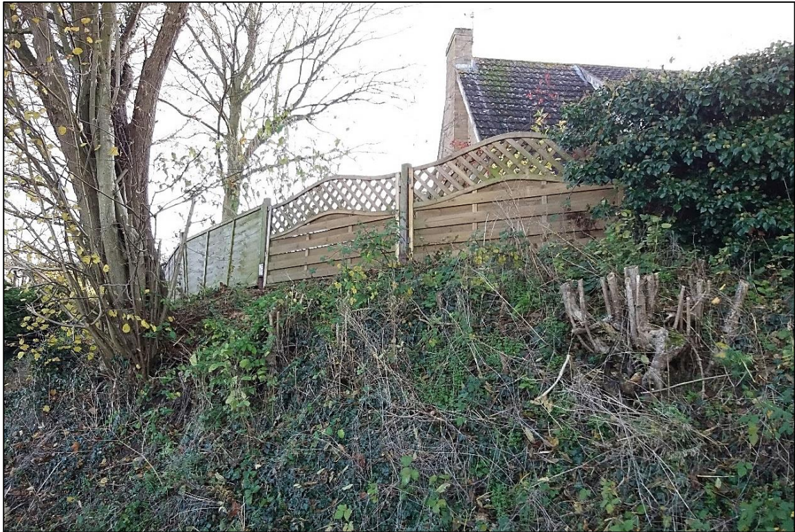
Panel and trellis fencing can also be inappropriate. In this case, it is imposing due to its high-level position, and its contrived character conflicts with the context of the area.
