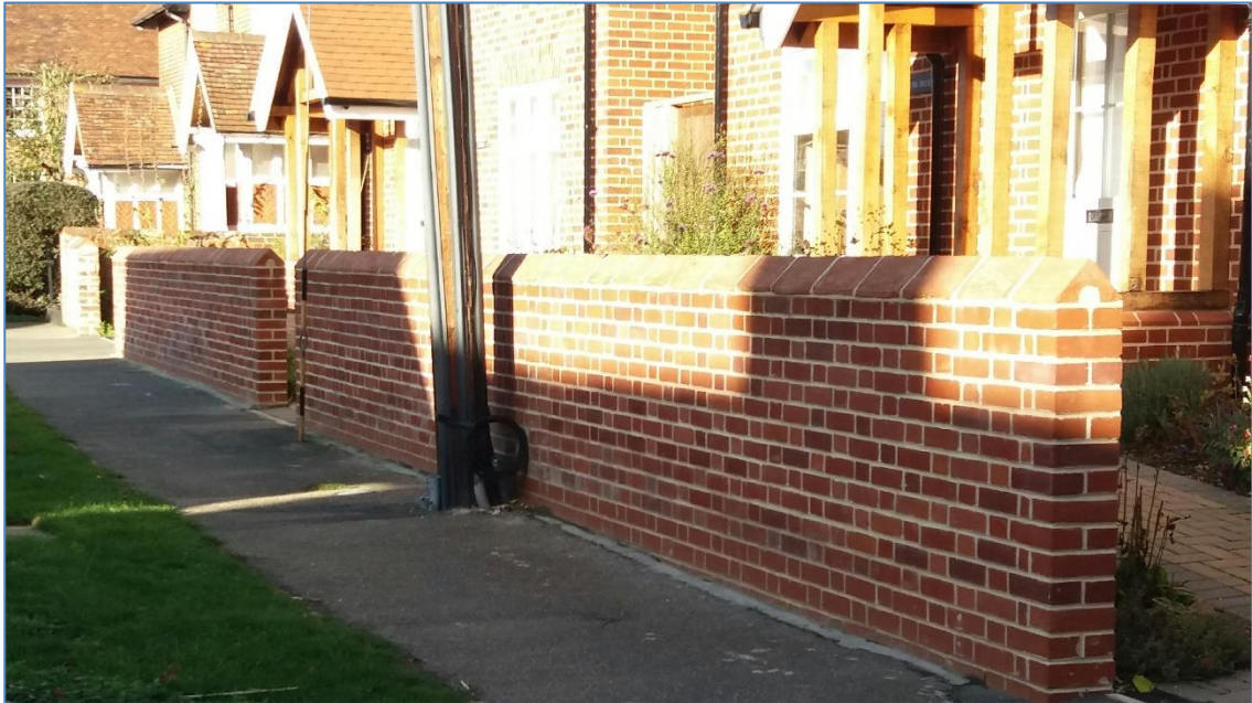
Good quality red brick boundary wall laid in Flemish bond, topped with purpose made coping bricks.
