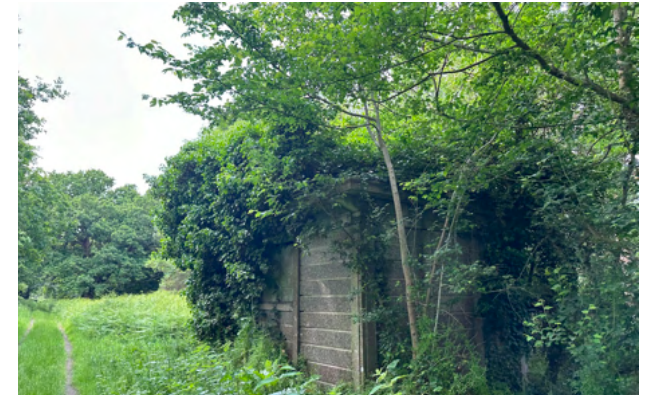
Plate 47 Former railway platelayer hut in a poor state of repair.
