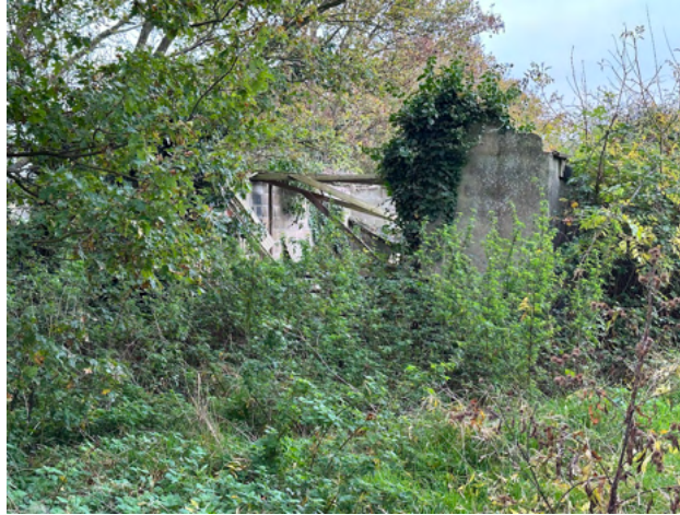
Plate 43 There are a number of scattered dilapidated buildings across the proposed conservation area that would benefit from repair and restoration work (here to the south west of Pond Hall).
