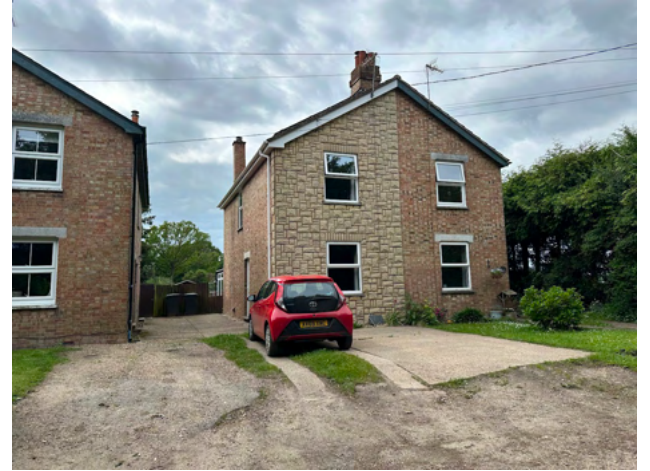
Plate 44 Inappropriate stone cladding to Falstaff Cottages.
